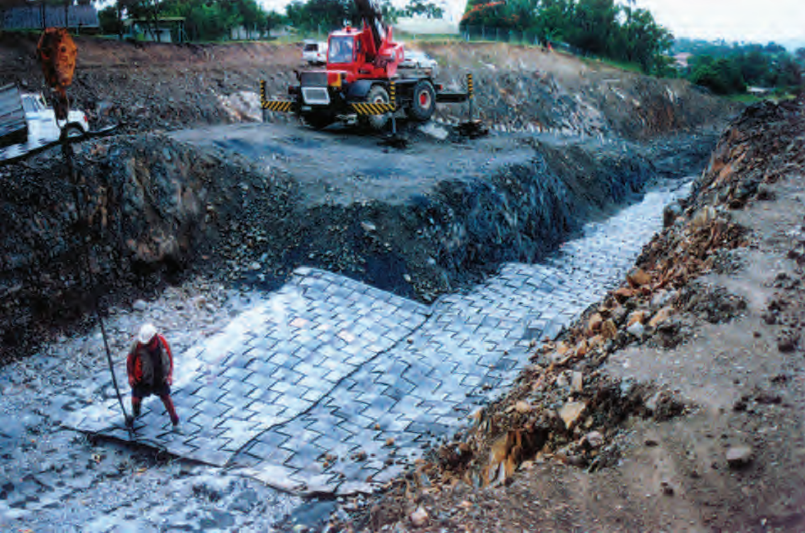
The picture shows Andromeda Blasting Mats each 7000 x 3000 x 30 mm being laid over a blast site on a railway cutting in the Brisbane area. (Leighton Project - photo by Zelman McLaren)
